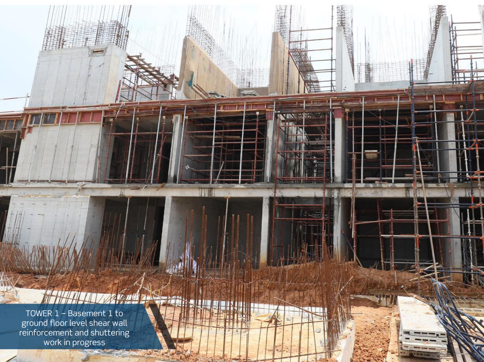
TOWER 1 – Basement 1 to ground floor level shear wall reinforcement and shuttering work in progress
